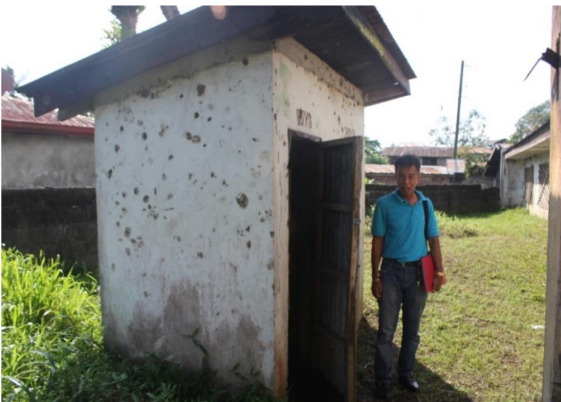
Figure 3. Inspection of a Typical Run-Down Toilet Facility in the Countryside. Photo by Josh Bahnarin Salud
