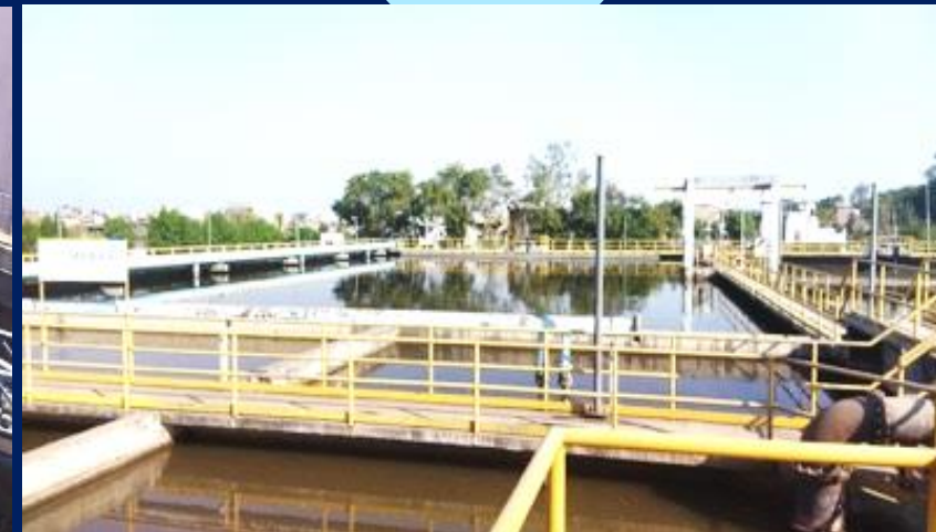
Sewage Treatment Plant
