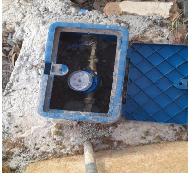
Figure A-4: A Jal Jeevan Mission water meter in Nagaraghatta village
