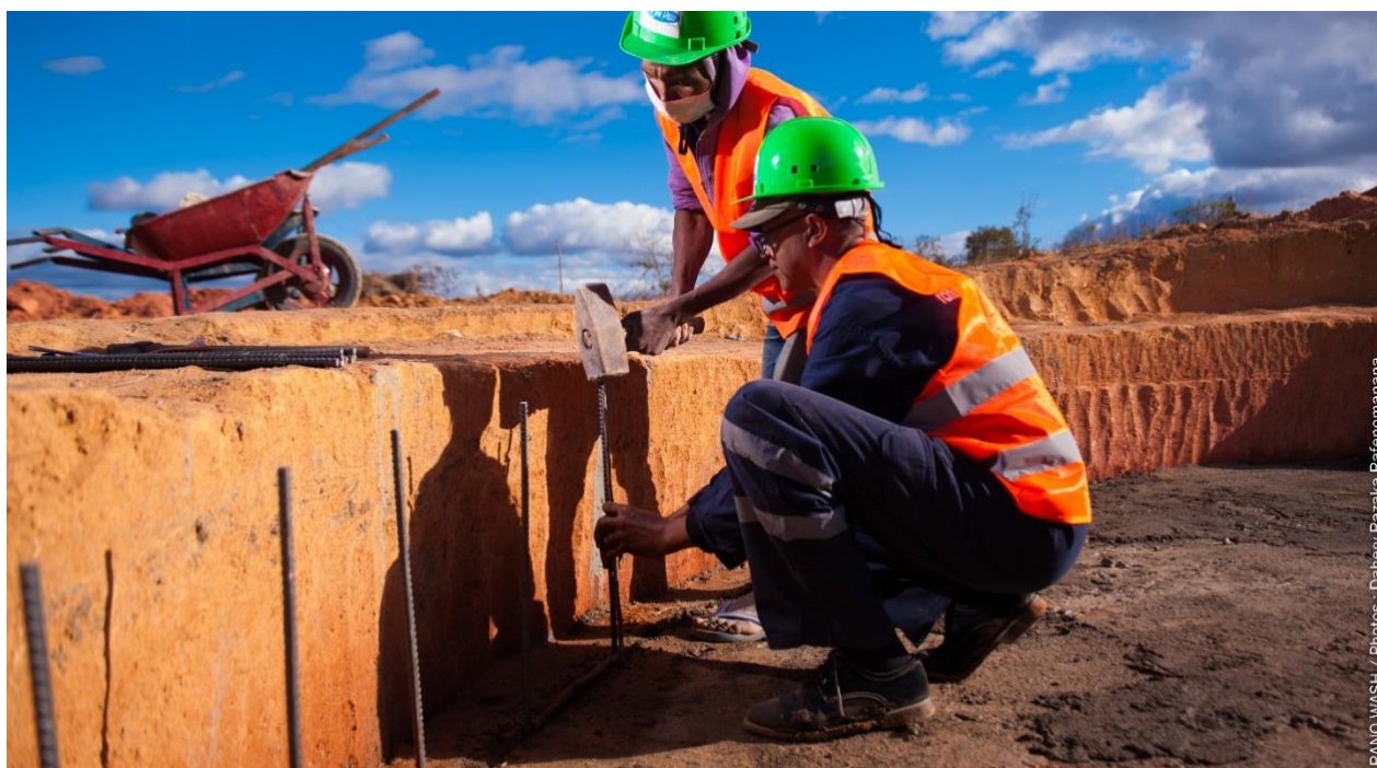
Picture 17. Workers from Lova Velu enterprise does a meticulous job in the installation of reinforcing bars, Morarano Chrome water system Alaotra Mangoro
