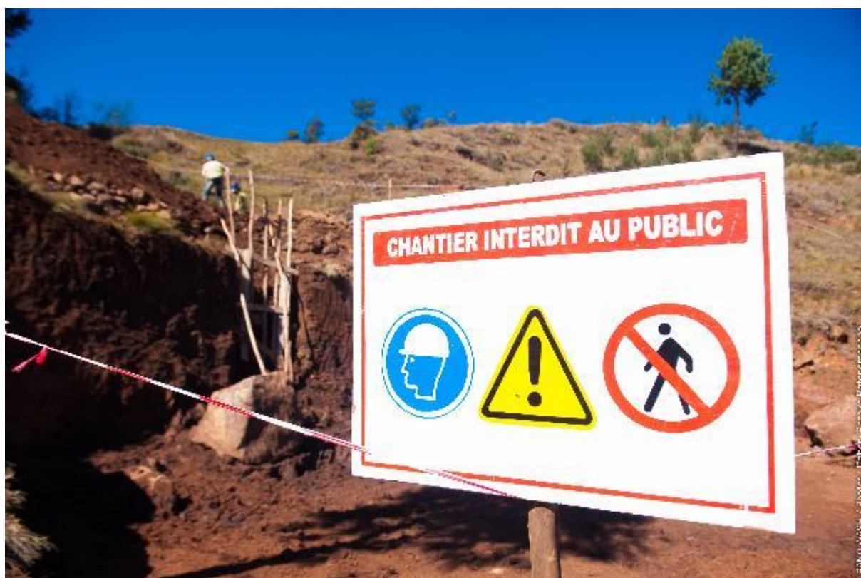
The photo above shows trenching work to install water supply pipes in the rural Commune of Antsoatany.
