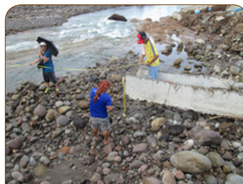
Diversion canal for Tombo ram pump damaged by Typhoon Haiyan
