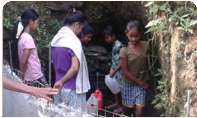
Women fetching water from the spring while construction of the impounding tank is ongoing
