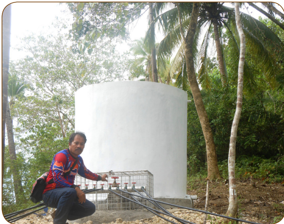
Green Empowerment Provincial Associate for Leyte, Rocky Peteros, kneels in front of a newly completed water reservoir in Brgy. Sto. Niño, Hilongos, Leyte. President Garcia, Matalom, Leyte.
