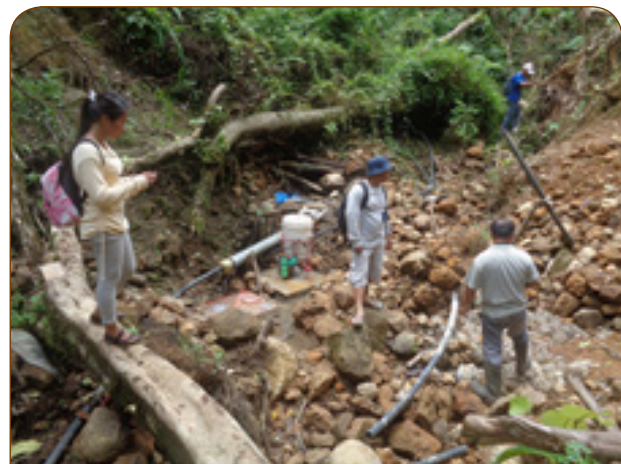
Lake Danao water system damage by earthquake
