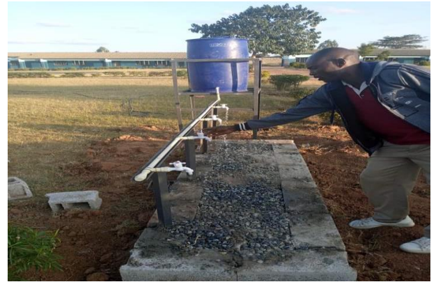
D. This is the prototype washing facility built around toilets (NB: The picture is from another District –MWANDI) and was used here for illustration purpose only)
