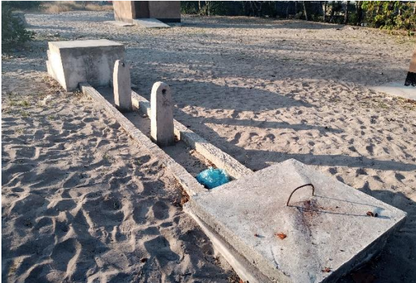
C. The Washing facility looks like it was vandalised, the WASH Coordinator indicated that it was yet to be completed after delivery of the drum.
