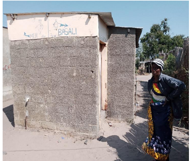
B. Abandoned Public toilet at Mandanga main Market
