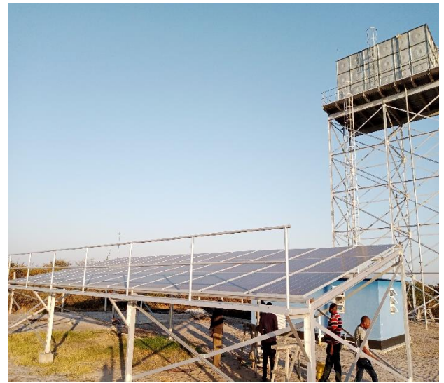
B. The Solar grid shelter comprising 36 solar panels to power the borehole pump and load into the 100m3 elevated Tank
