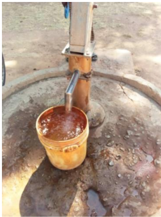
FIGURE 36. RUST-STAINED BUCKET FROM HAND PUMP WATER IN LUNTE
