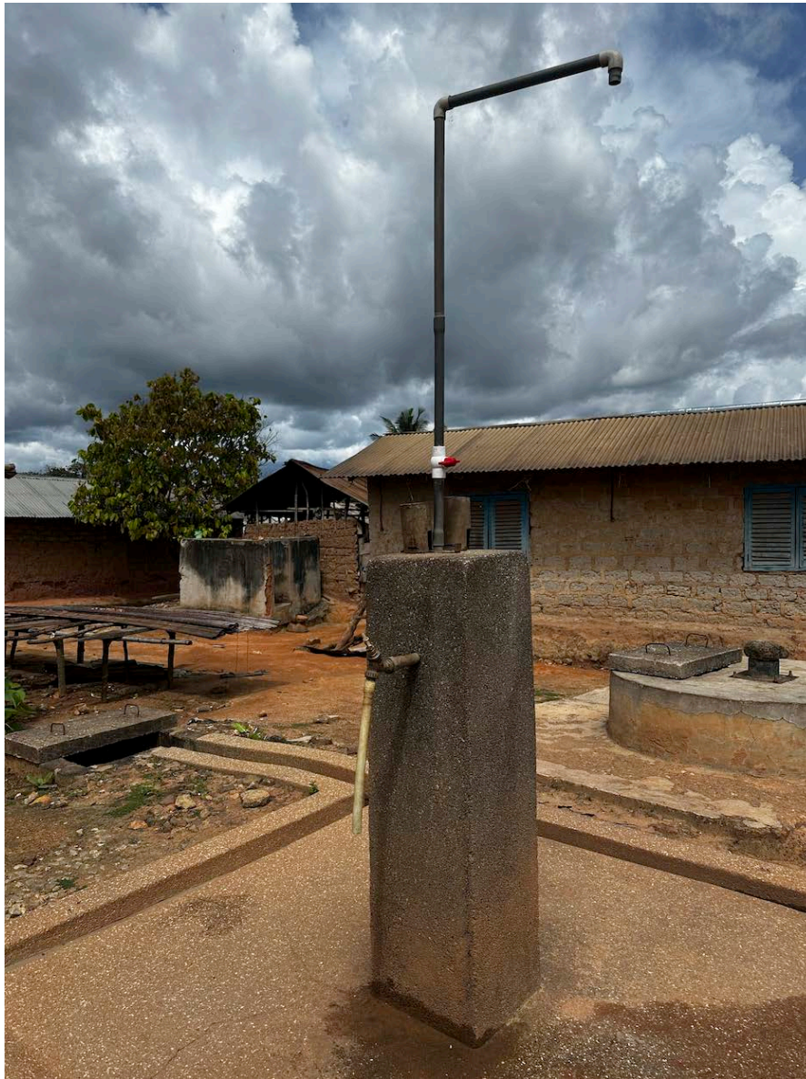
Figure 4. Tapstand in a rural village in the Asutifi North District in Ghana (Source: The Aquaya Institute)
